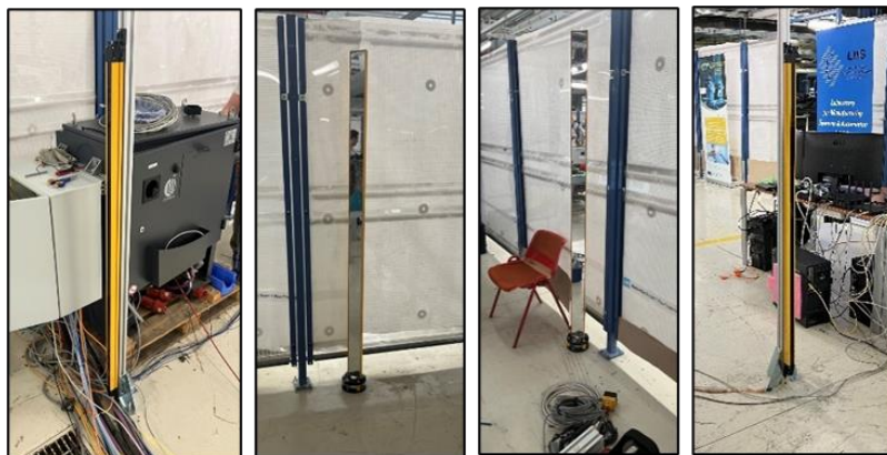
Figure 34: Safety light barriers and mirrors
