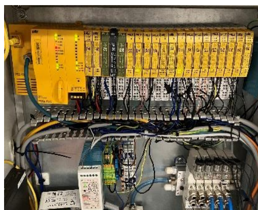
Figure 37: Safety PLC integration
