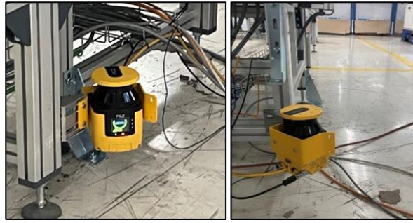
Figure 35: Safety laser scanners installation
