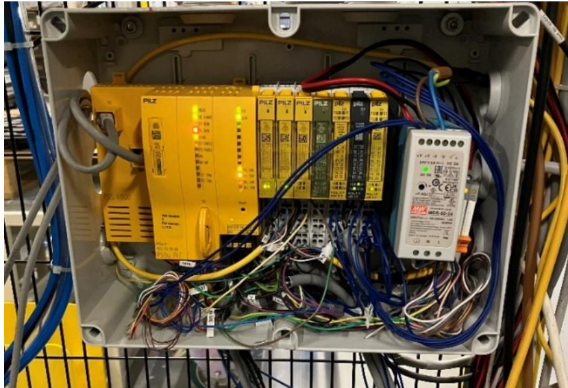
Figure 115: Safety PLC integration
