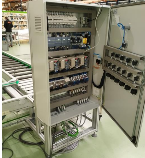
Figure 4: Conveyor Electric and communication cabinet
