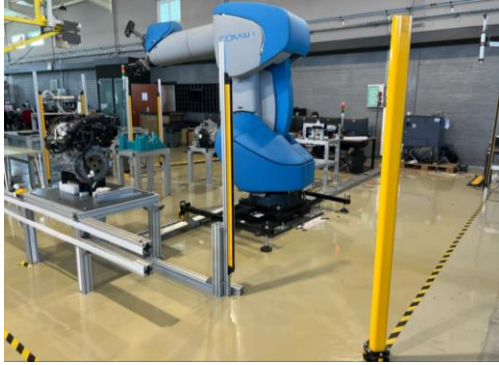
Figure 25: Light Barriers installed at LMS Automotive Small-Scale Pilot
