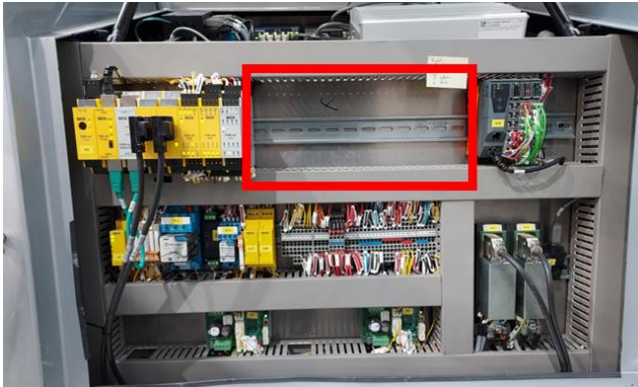
Figure 41: Place for SICK IO modules and PILZ safety PLC
